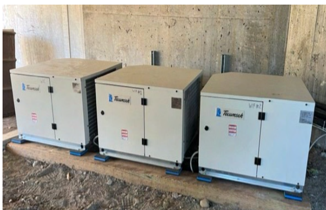
Outdoor cooling system for the kitchen
